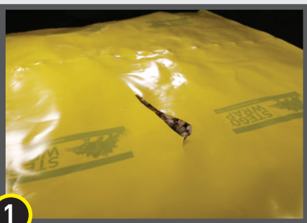
1 Occasionally there are larger holes in the vapor barrier that require a patch.
