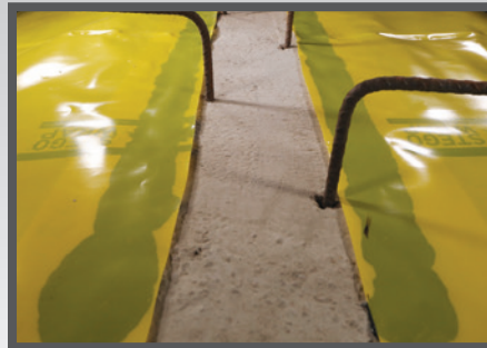
Onto Interior Grade Beams at Impediments: Seal Stego Wrap to concrete with Stego Mastic.
