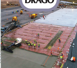
VAPOR INTRUSION BARRIER
