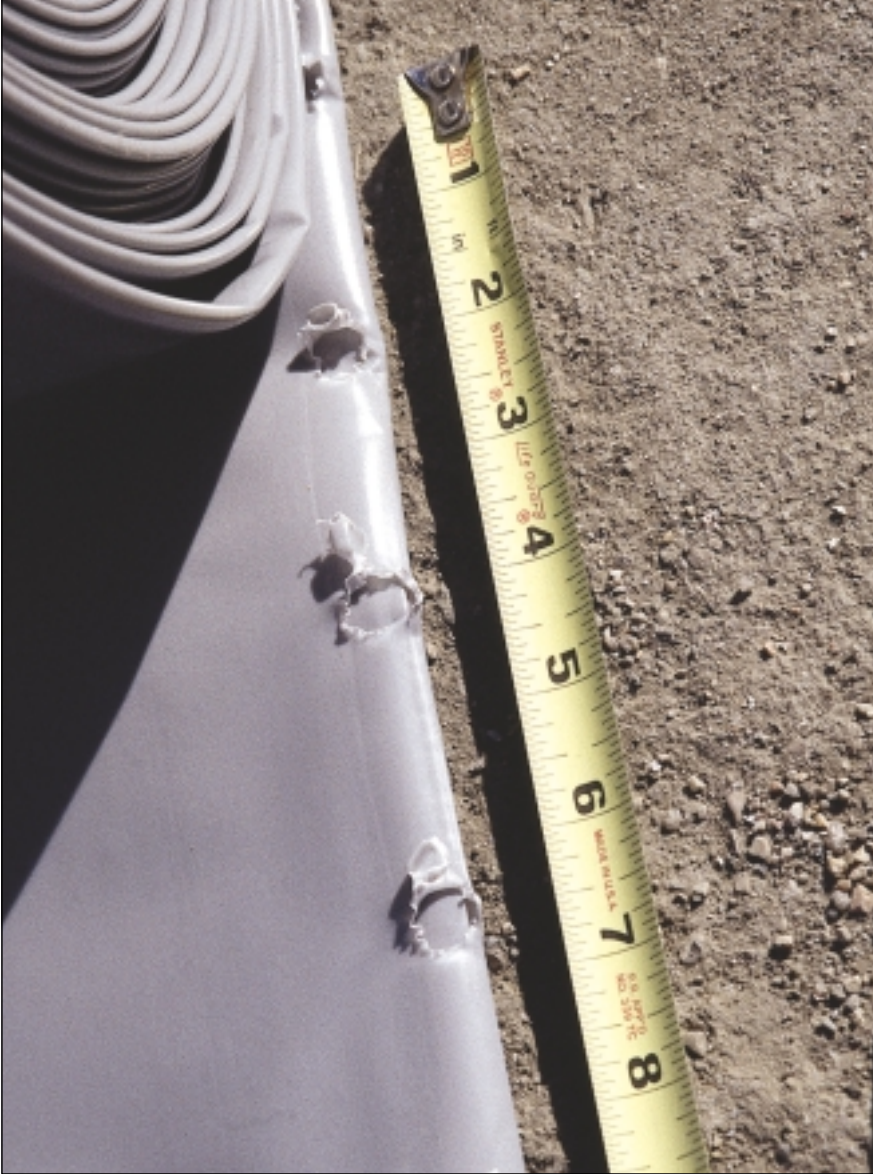
Left: This vapor barrier had been damaged before it was placed on the subbase. Below: Visual examination revealed the number of punctures caused by compacting granular fill on top of a vapor retarder.
