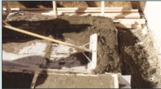
Before examining the vapor retarder for punctures, we carefully removed the fill with a broom.
